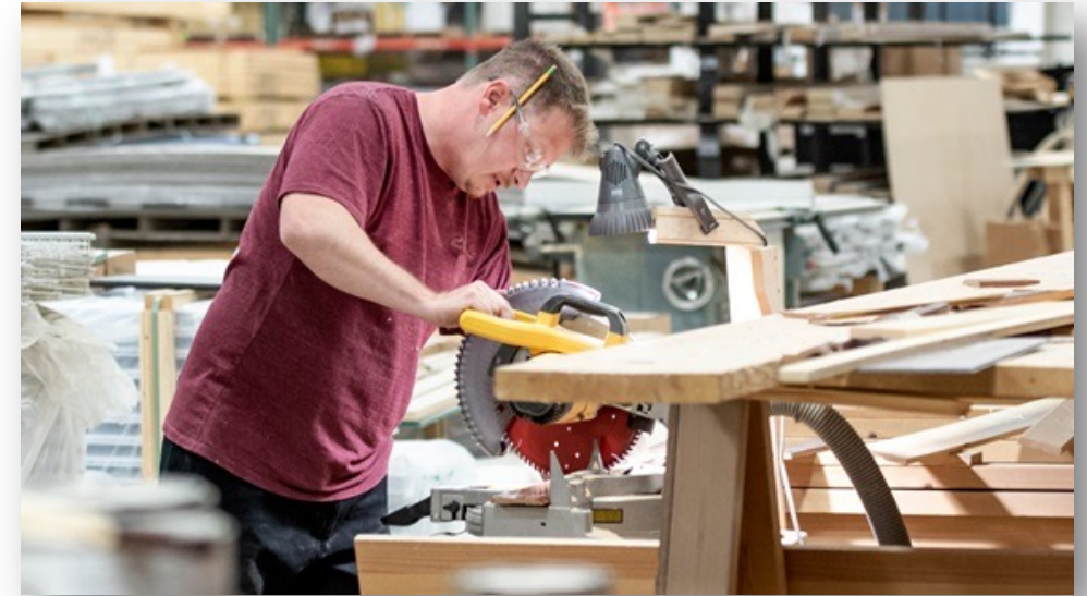
A worker cuts lumber at Dynamic Homes, a modular-construction firm in Detroit Lakes, Minn. Image courtesy of Ho-Chunk Inc.
